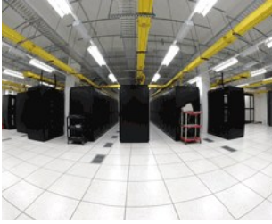
Our Tier 1 East Coast Data Center provides our clients with Disaster Recovery, Testing, Remote Access as well as Private Cloud Capabilities
